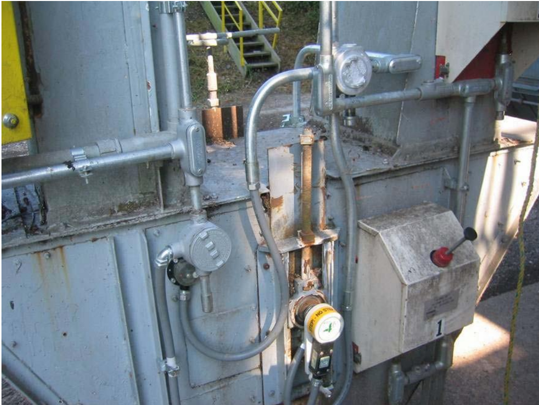
Figure 36: A bucket elevator boot with installed hazard monitoring sensors and conduit low point drains. (Photograph courtesy of 4B Components, Ltd.)
