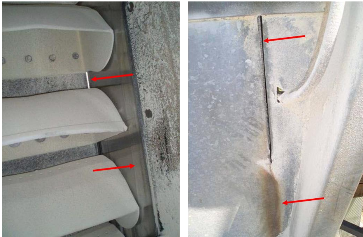
Figure 16: Inside elevator (left) and outside elevator (right) showing discoloration and slits in steel casing from the effects of friction and wear due to severe belt misalignment. (Photographs courtesy of 4B Components, Ltd)
