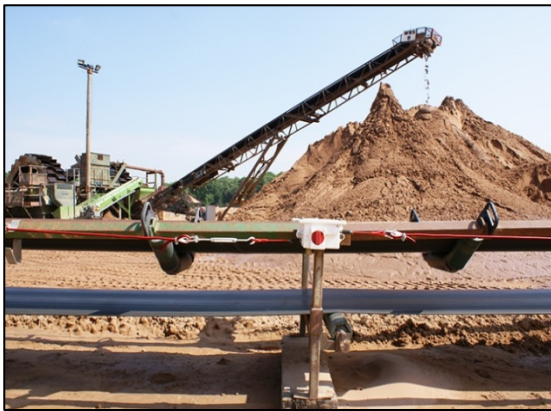
Pullswitch Installed on Open Conveyor at Sand and Gravel Facility
