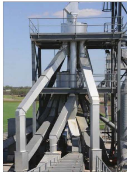
Modified Rapat distributor with enlarged spouting (middle platform) below a second, new Rapat distributor (top platform). Photo by Tucker Scharfenberg.
