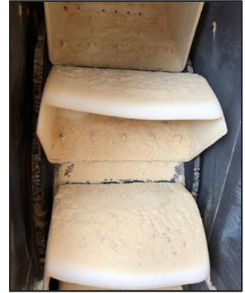
Elevator Buckets with Extensive Wear
