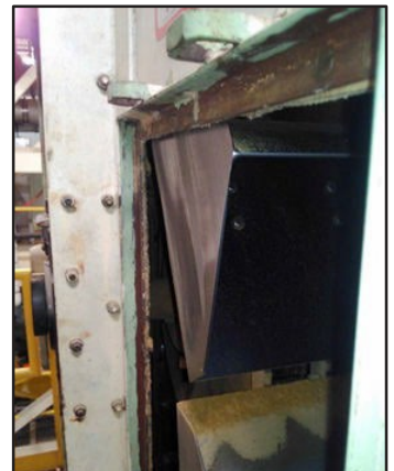
Steel Bucket Rubbing Against the Elevator Casing
