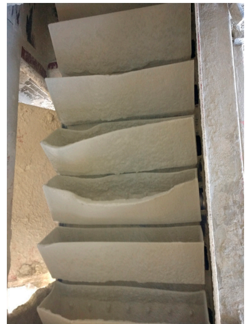
Metal buckets distorted and broken
