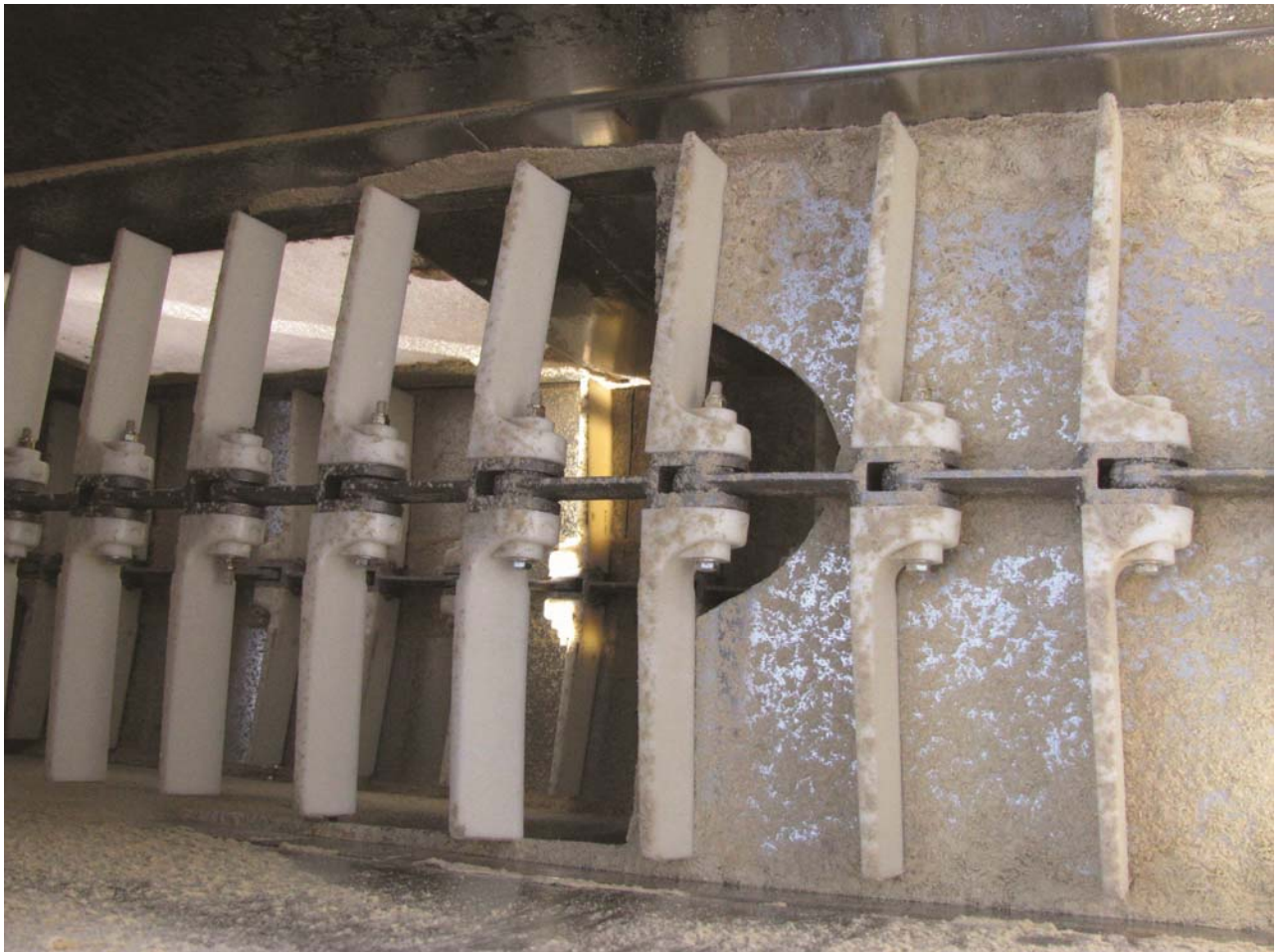
Bolt 'n' Go chain system running on conveyor
